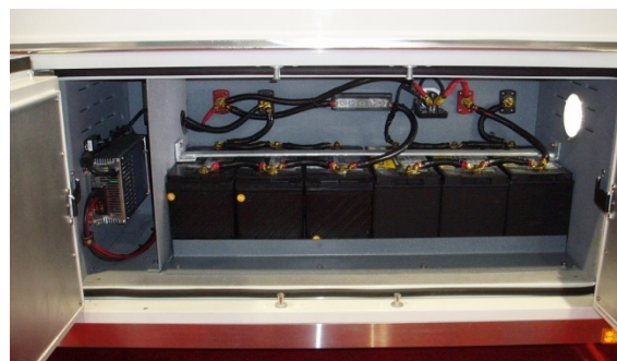
Exterior battery compartment with 90-amp battery conditioner.
